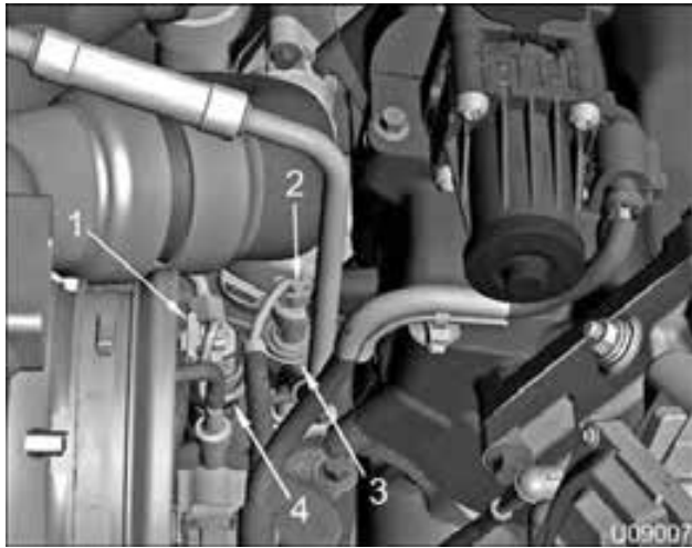
Figure 121 EOT sensor and EOP sensor
